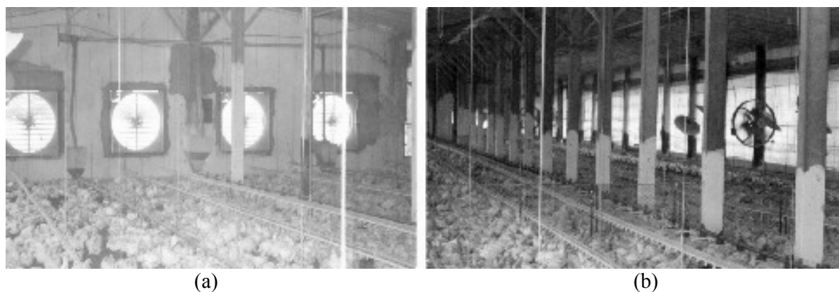
Figure 1. View of the exhausting fans (a) inside G2, and axial fans and side curtains (b) inside G1.
